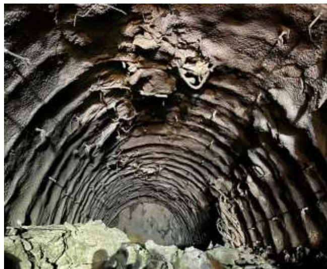
Figure. 5: Deformation of Lattice Girder along crown centerline
