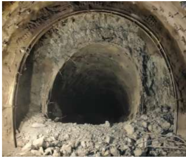
Figure. 2: Extreme squeezing at Tunnel No. 10 (SRRP)
